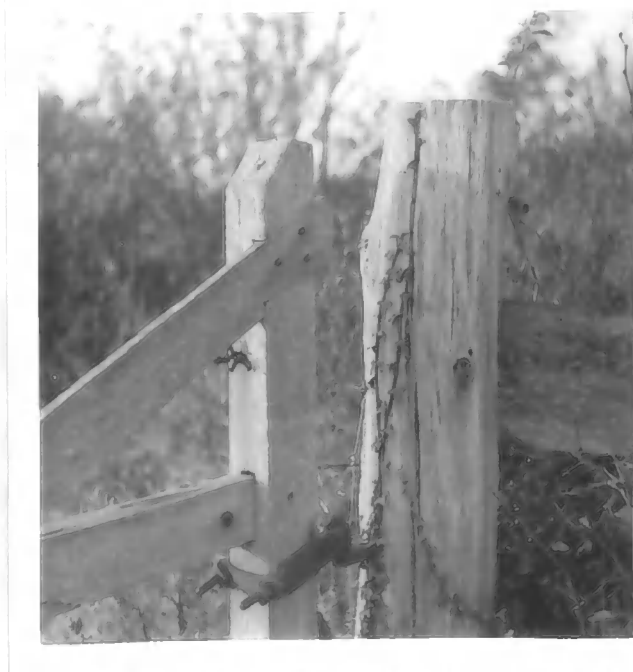
Plate 22. Detail of Harr of the above, showing method of construction. Photograph:- T. E. Morland.
