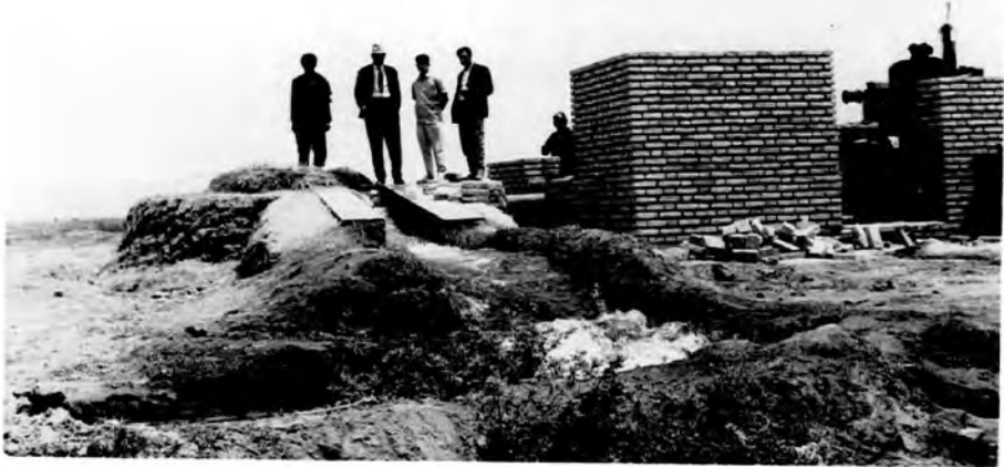
The final stage of a new electrically powered pump and its building on the Khiaban complex.
