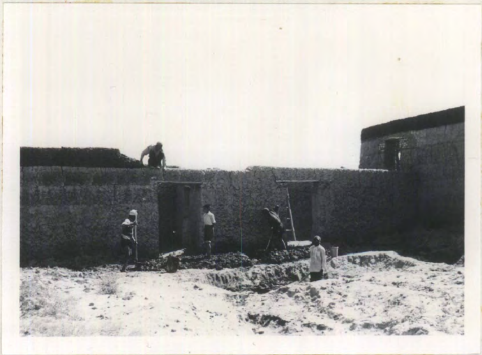
Haji Nasir - wall being constructed in courses by a party of village workmen.
