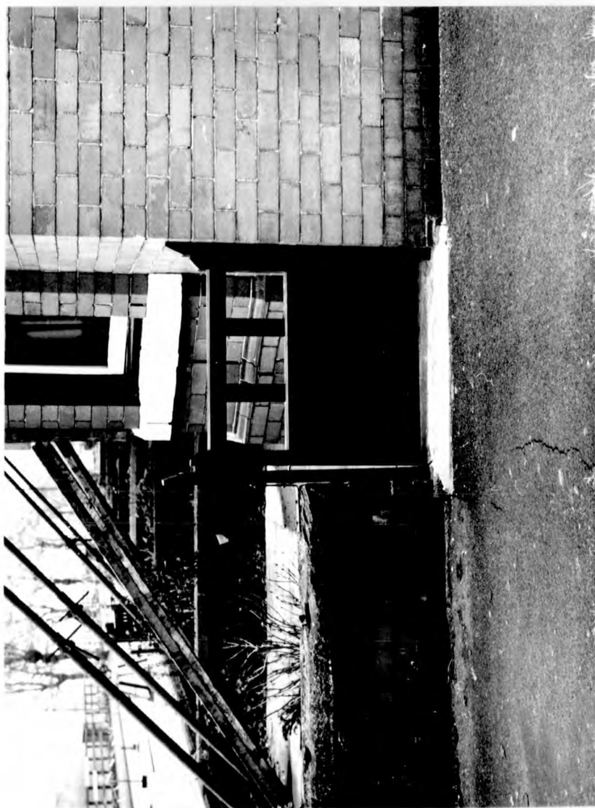
PLATE 6.2 STRUCTURAL DAMAGE AT SECTION B
