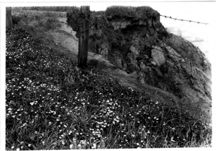
Plate IX: Cliff top recession north of Tunstall Hope is rapid, owing to the lack of cohesion of the superficial deposits which readily fall on to the beach, and to the general shortage of beach material which allows the waves to attack the cliffs strongly.
