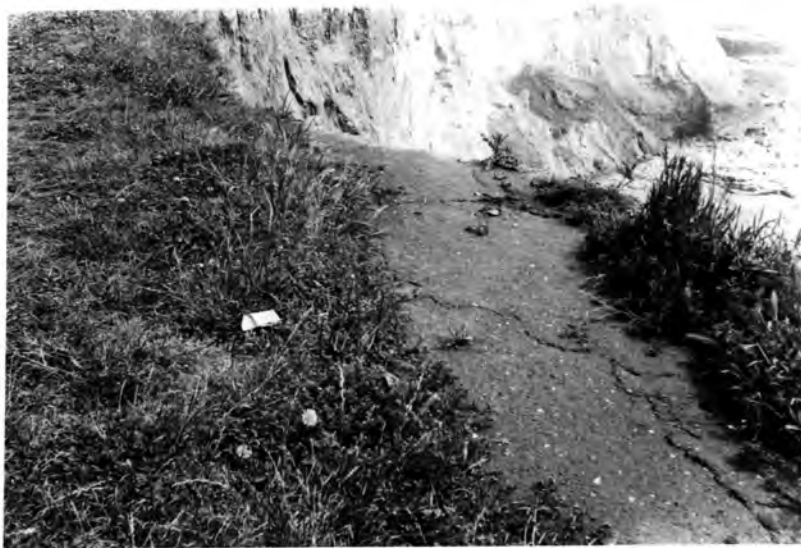
Plate XIV: Salterfen Point from the south. The resistant yellow bedded limestone is covered by a layer of less resistant boulder clay, which is covered by sandy deposits displaying bedding. Cliff top recession is rapid, and the footpath in the foreground has been partly washed away.
