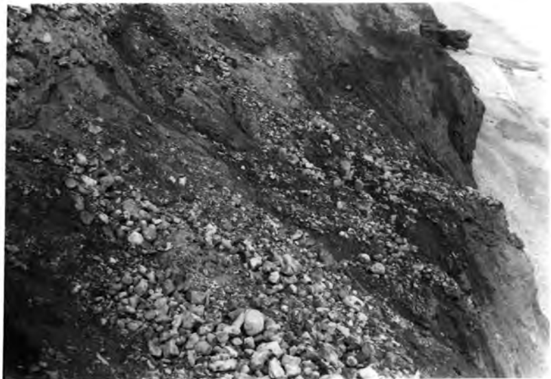
Plate VI: South of Tunstall Hope the gravels and sands associated with the Tunstall overflow channel form an important part of the sea cliffs. These superficial deposits suffer from atmospheric as well as marine denudation. The large boulders fall when the supporting pebbles are washed away by rain wash, and they tend to accumulate on the top of the boulder clay.
