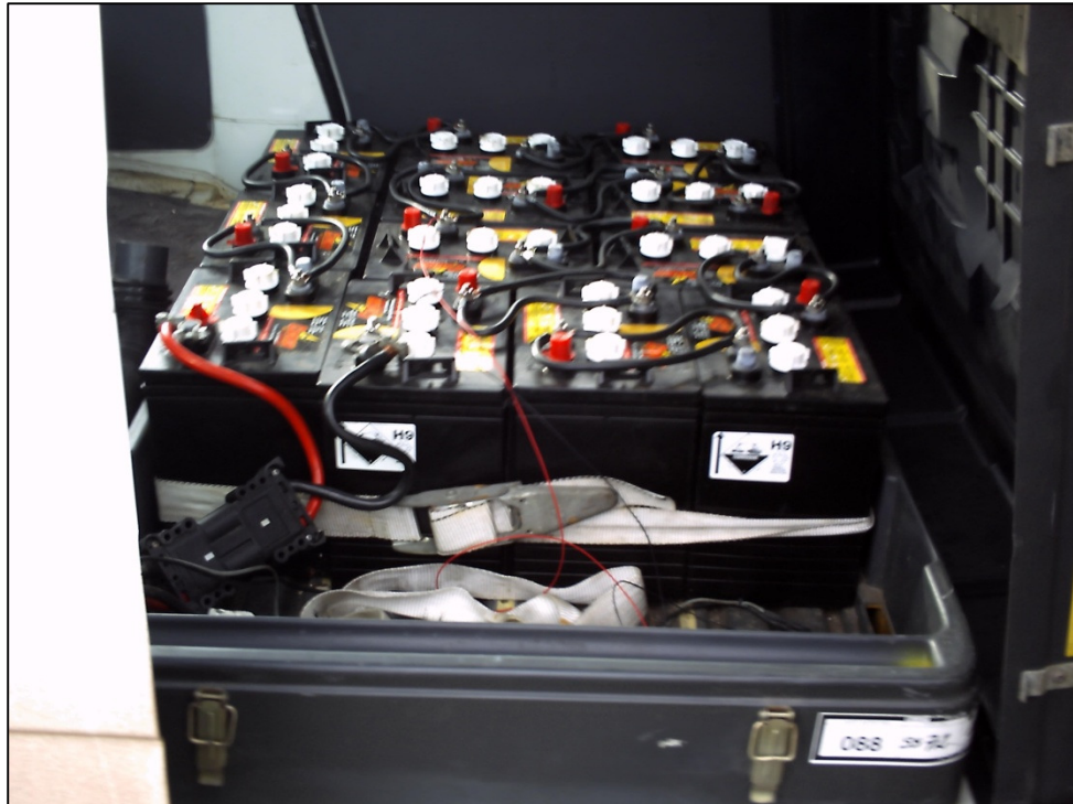
Fig 6.1 - The battery pack in John L's Elcat van showing 12 lead-acid batteries in series. All the batteries are located in the same place, in a standard battery box behind the front seats. A lid goes on to the box so the van can be used for carrying cargo. You have to climb over the box to get to the back seats.
