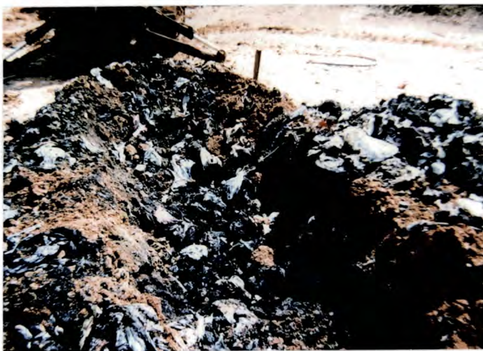
Fig. 1.6 A close-up of GDB landfill cover with the soil partially removed. The remain of waste, after embedded for about 10 yr, is mainly plastics, with the organics degraded. The cover was dug for lying water pipes and cables.
