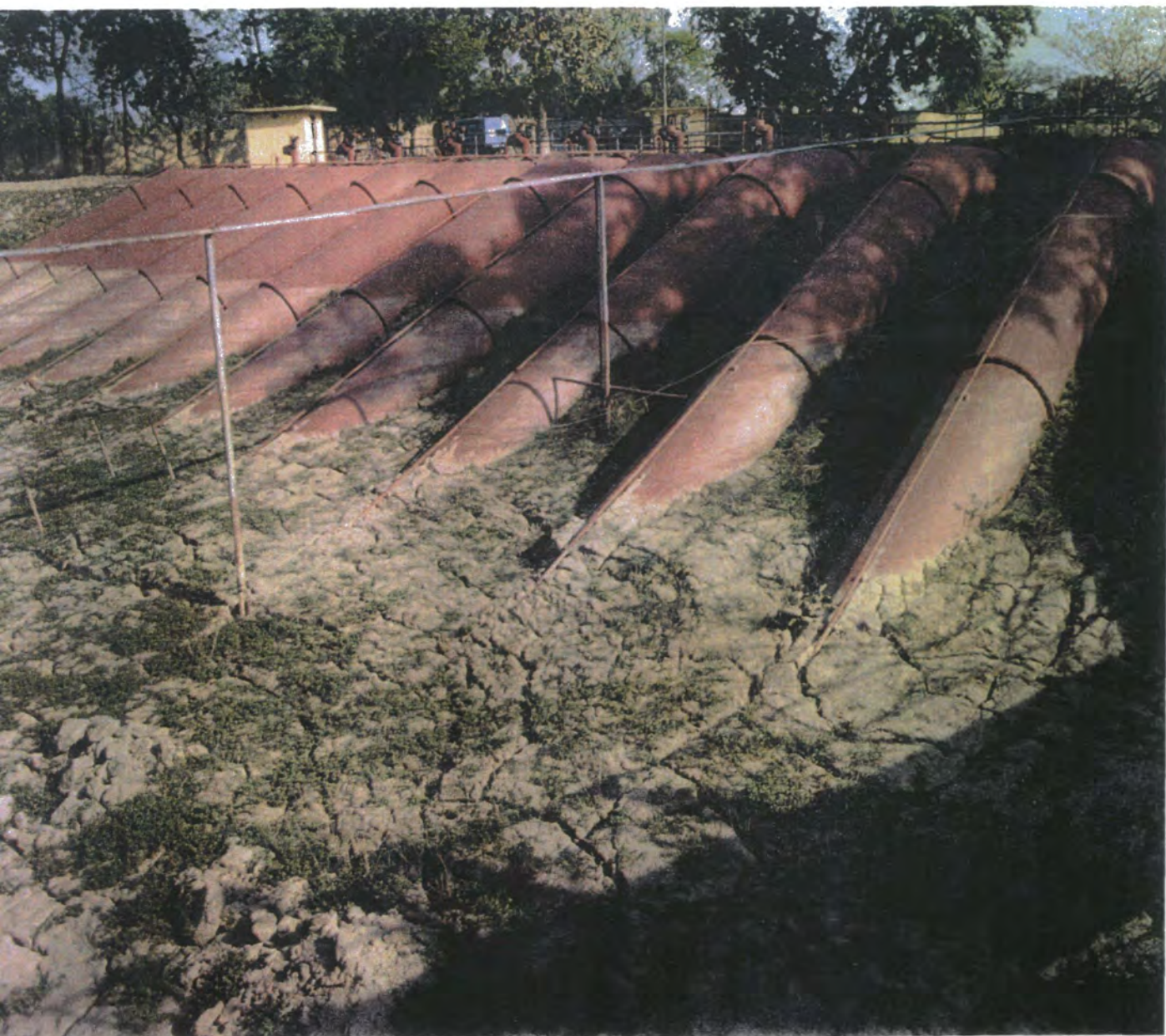
Photograph 5 Another view of the Ganga: Kabadak pump house in the dry season
