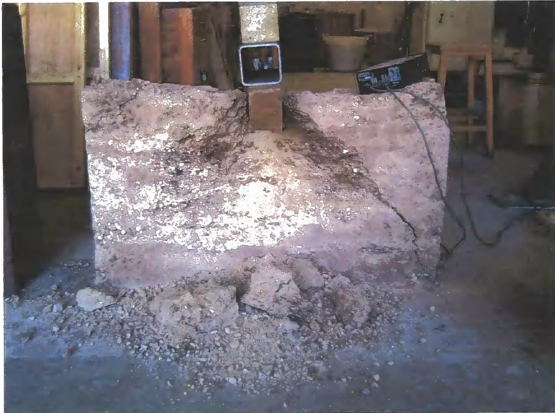
Figure 2.20 Wall 1 diagonal shear and out-of-plane failure
