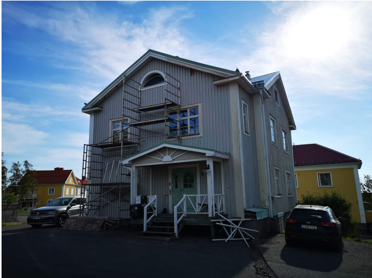
Figure 26: Scaffolding denoting repair work on former apartment house. Photo by author, August 2022
