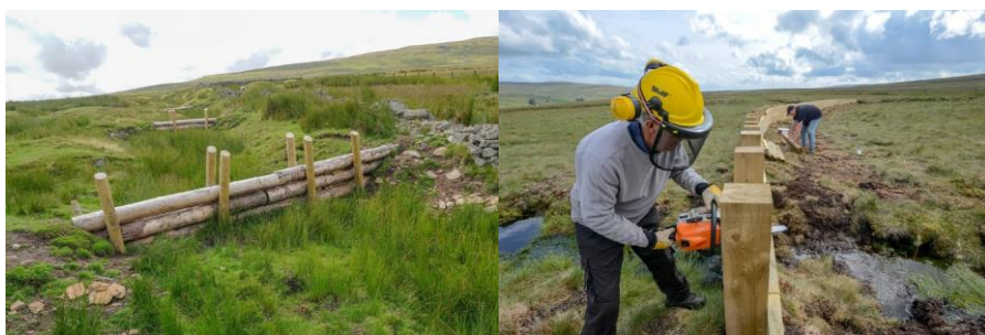
Figure 3. Example of a leaky barrier (left) and a timber fence (right) installed on the Killhope Burn in upper Weardale (Photograph taken from Environment Agency et al., 2021).
