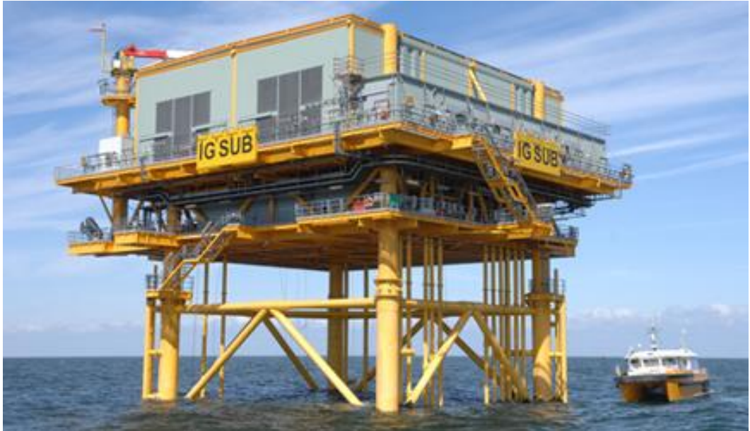
Figure 30: Example of a Fixed Substation Installation at Horns Rev Wind Farm
