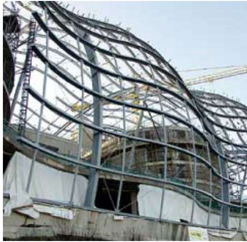
Figure 1.6 - Frame of the outer skin of the sage building, on which cladding is mounted surrounding the concert halls
