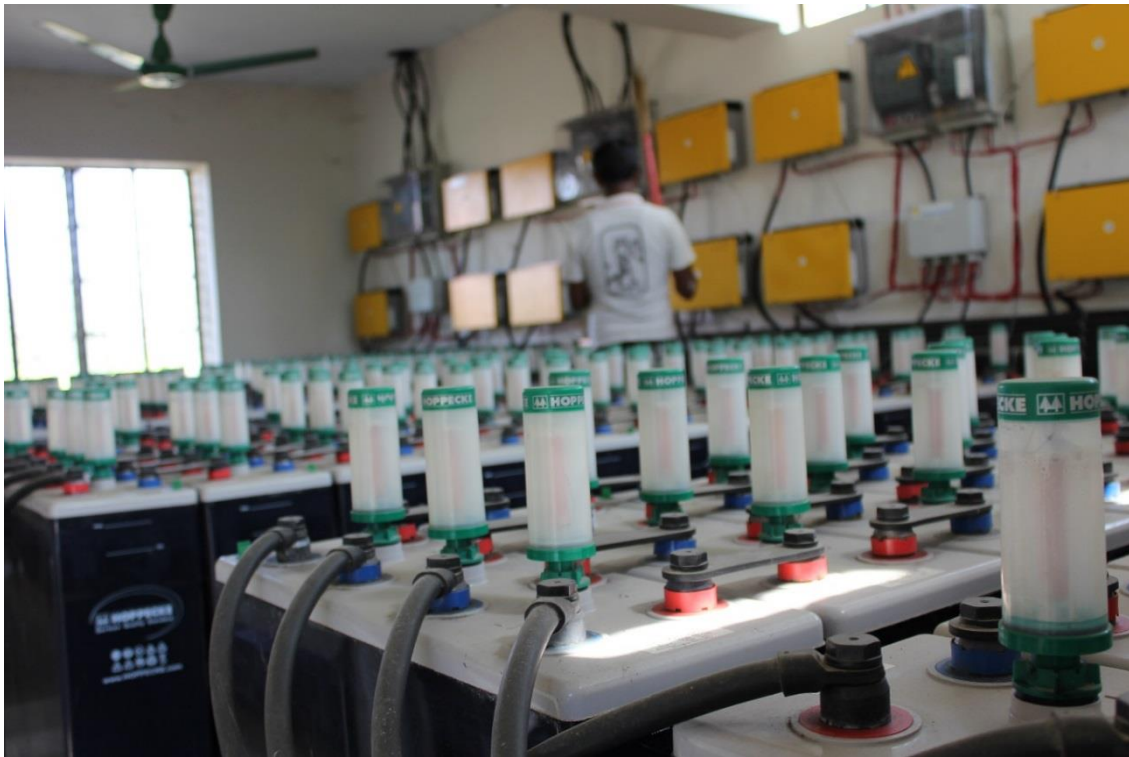
Figure 6:11 Inside Purobi mini grid power station
