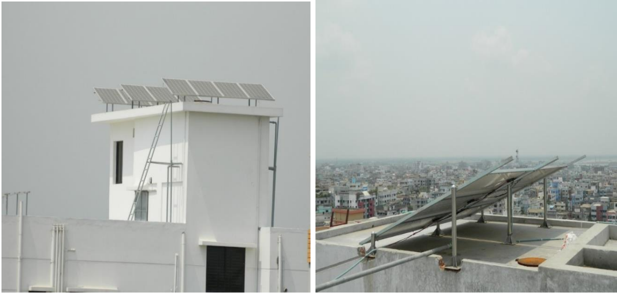
Figure 8:4 Solar panels on water tanks Source: Author
