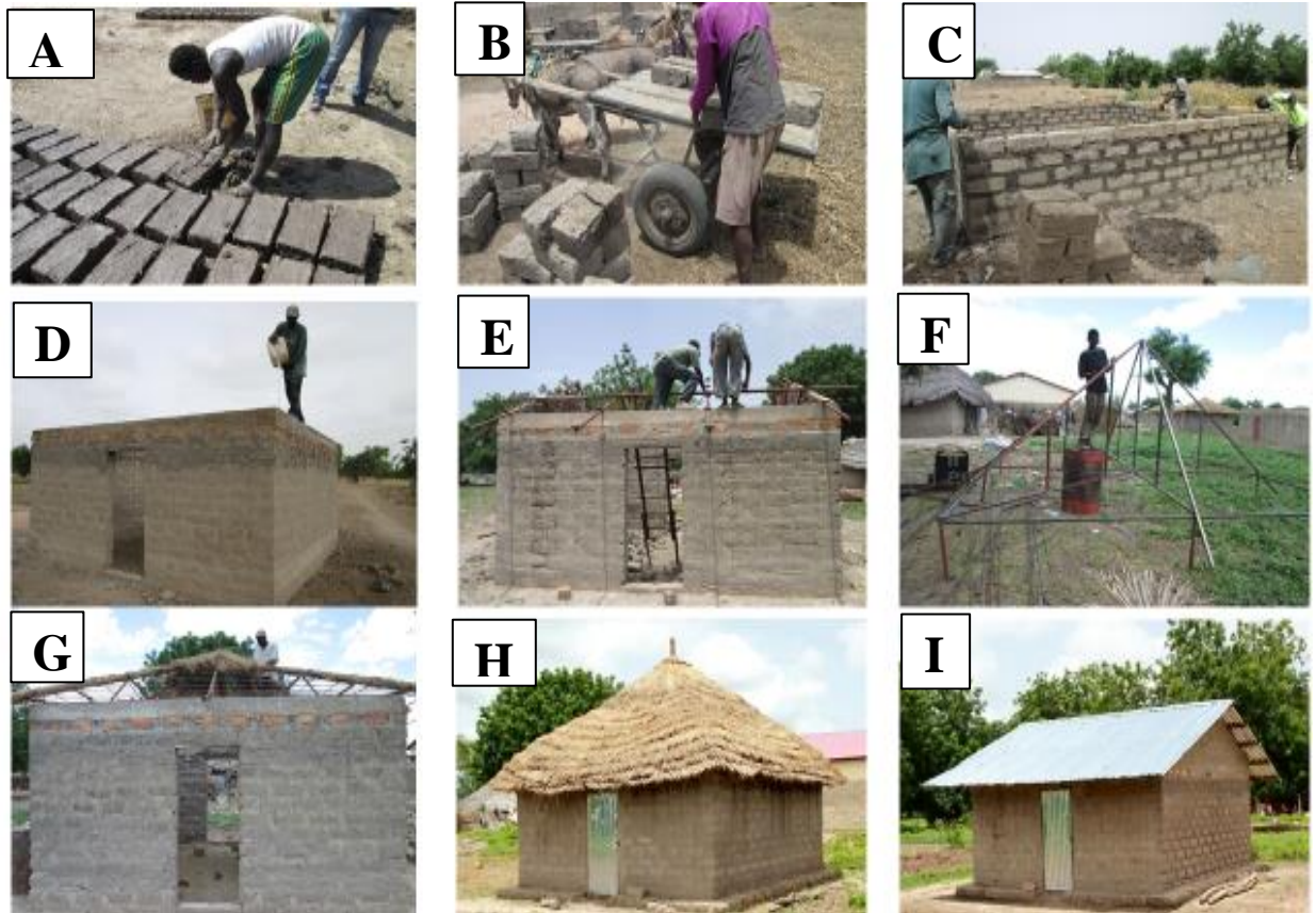
Fig. 2.3: Experimental houses under construction: A) mud blocks being sun dried, B) block transportation, C) wall construction, D) wetting concrete lining, E) attaching wood to metal frame, F) assembling metal roof frame, G) putting thatch on roof frame, H) complete thatch roofed house, I) complete metal roofed house
