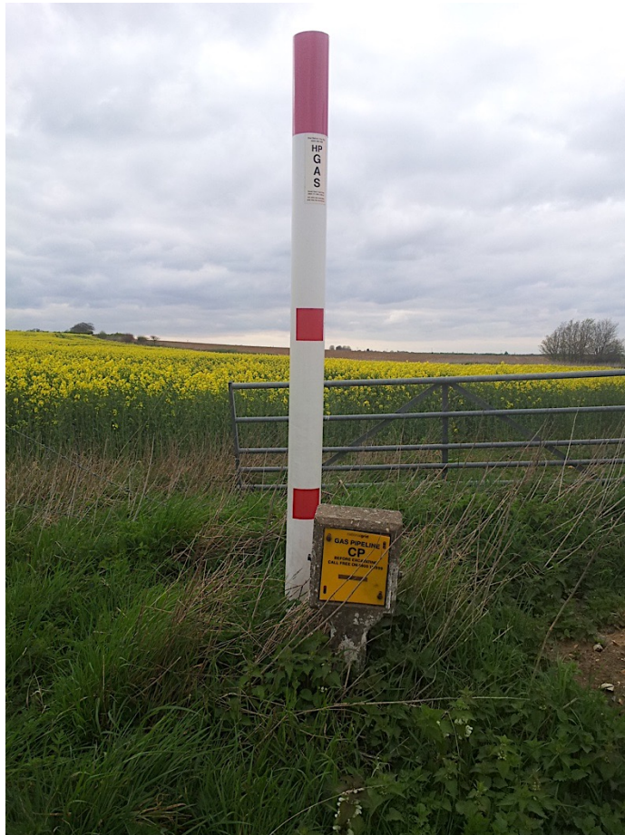
Figure 17 - Photograph of NTS pipeline marker in Norfolk, 2014
