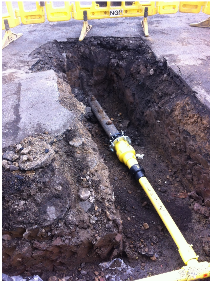
Figure 18 - Photograph of a distribution pipe in Middlesbrough, 2015
