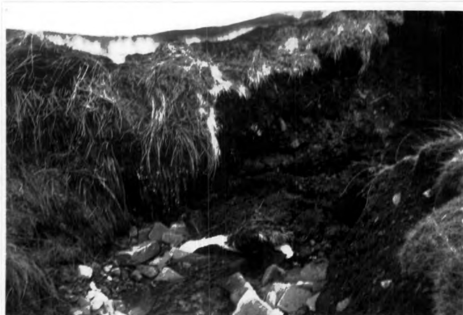
The saturated peat and the severe frost effect on the vegetation cover
